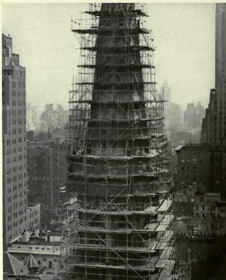
Steel pipe serves a structural purpose in the scaffolding erected for the repair of a cathedral spire in New York.
